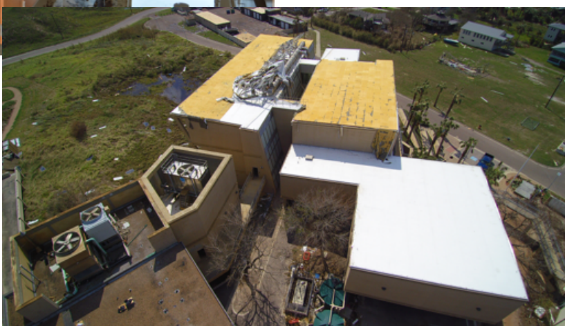
High winds tore solar panels from the roof of the Institute, causing flooding throughout all 3 floors of labs and offices.
